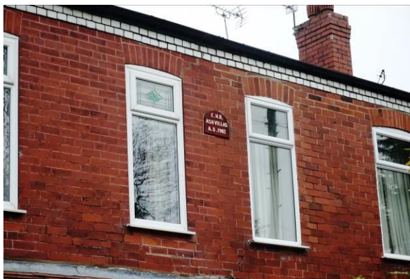
Inappropriate uPVC replacement windows and modern stained glass detailing at Ash Villas (east side)
