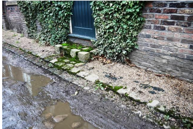
Traditional road and pavement surfaces, in a poor condition
